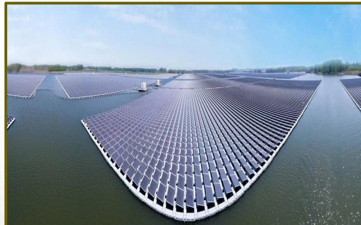
Hunan Floating Power Station 50MWp
